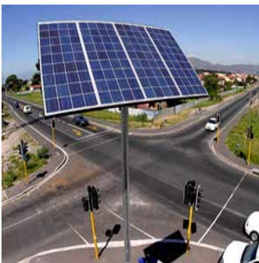
Solar powered traffic lights
