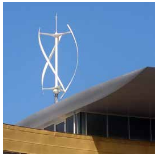
Roof-mounted wind turbine
